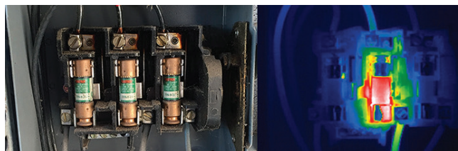
Thermal Image, Corroded Fuse
